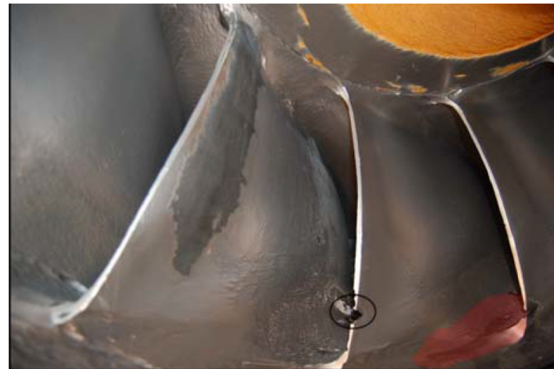
Erosion at pressure side of blade
